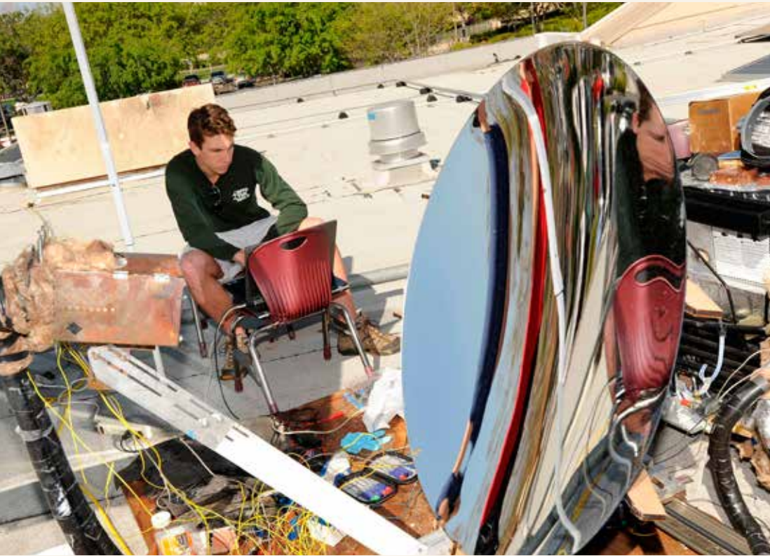
On the roof working on a solar-powered absorption chiller or in the dance studio perfecting his technique, Coulter exemplifies Santa Clara's goal of educating the whole person.
